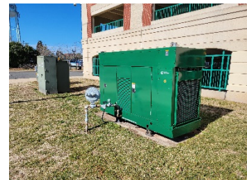
Overhauled emergency generator returned to Manassas parking garage
