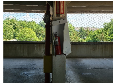
Damaged fire extinguisher cabinet at Woodbridge station parking garage
