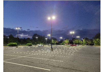
New LED lighting at Fredericksburg.
