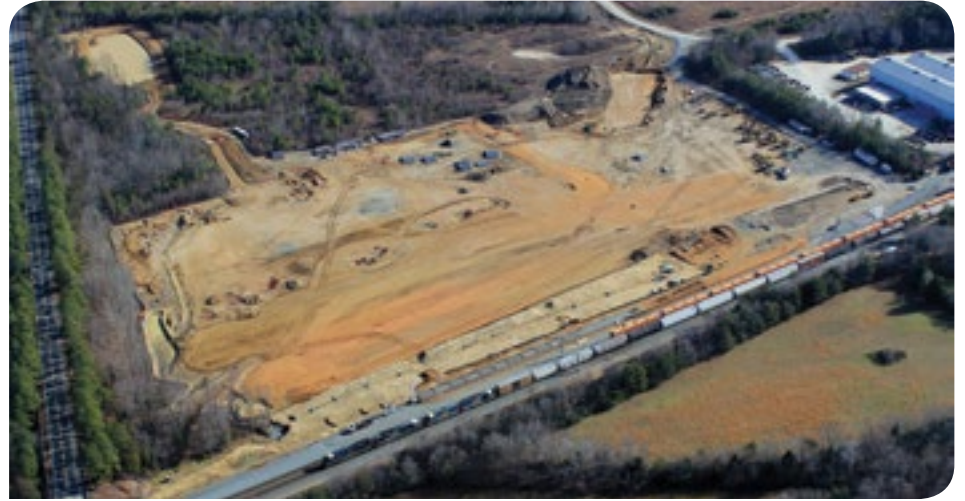
▲ CSXT freight trains run past the worksite for the new Spotsylvania Station. VRE's contractor is working on new track and platforms in the foreground, while the County's contractor works on fill and drainage for the parking lot.
